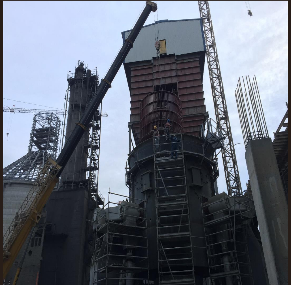
CEMENT MİLL MVR 5000 C4 ESKİŞEHİR CEMENT PLANT ESKİŞEHİR / TURKEY 2017
