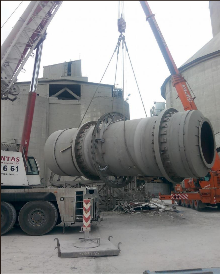
ROTARY COOLER ESKİŞEHİR CEMENT PLANT ESKİŞEHİR / TURKEY 2017
